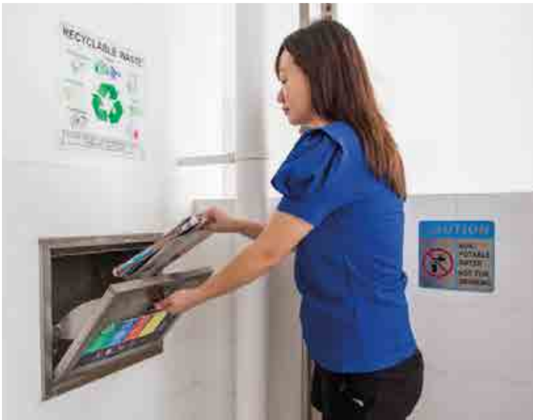
Separate chutes for recyclable waste
