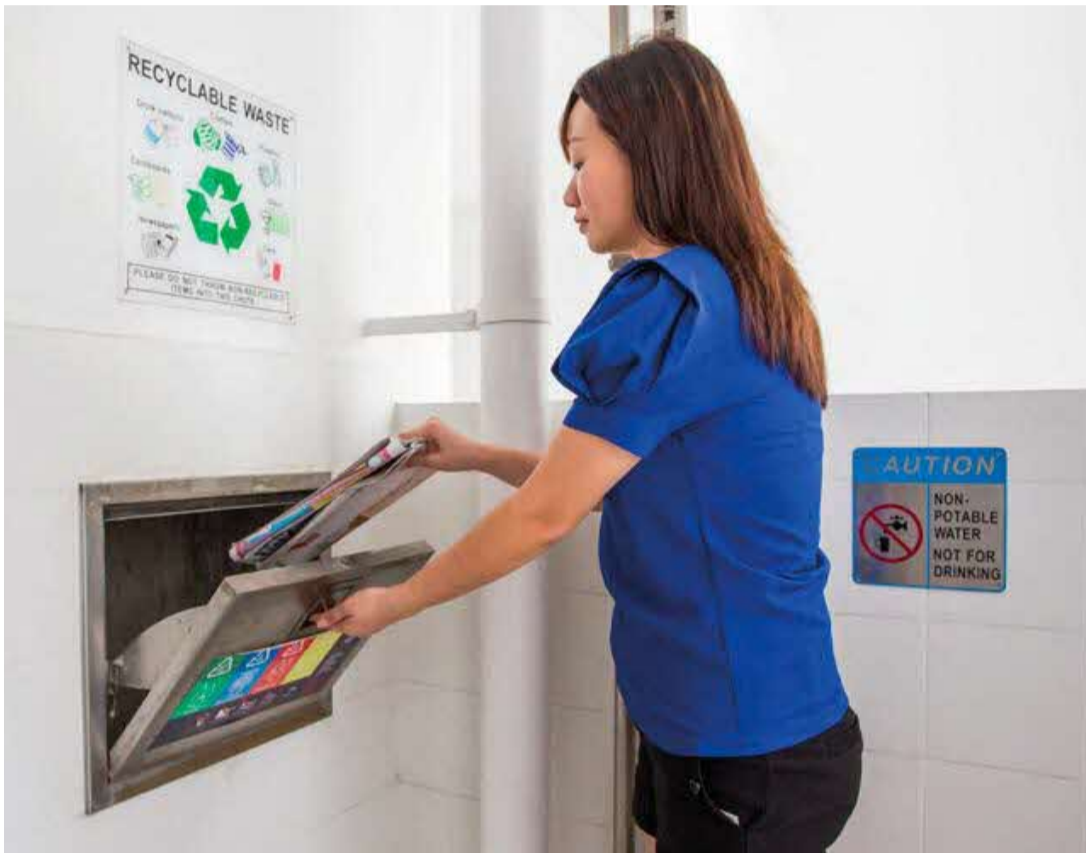
Separate chutes for recyclable waste
