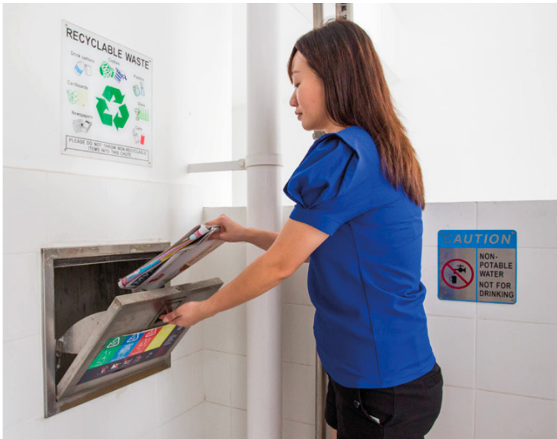
Separate chutes for recyclable waste
